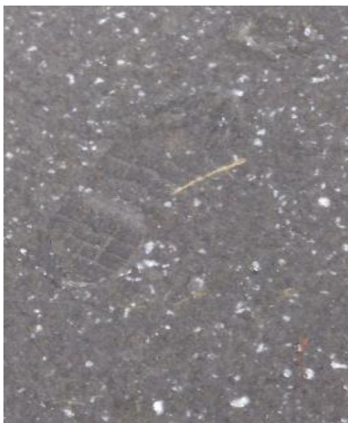
Plate 7.2-Brittania Greenway asphalt section in sub-zero temperatures showing ice
